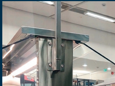
Power supply from ceiling
