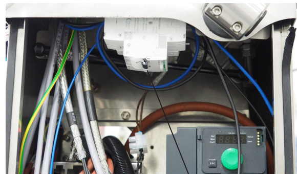
Earth leakage circuit breaker test button
