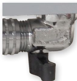
1. Control valve of steam jacket
